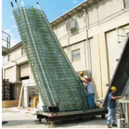
(Right Photo) Inclined, voided, precast concrete column being handled in the casting yard.
