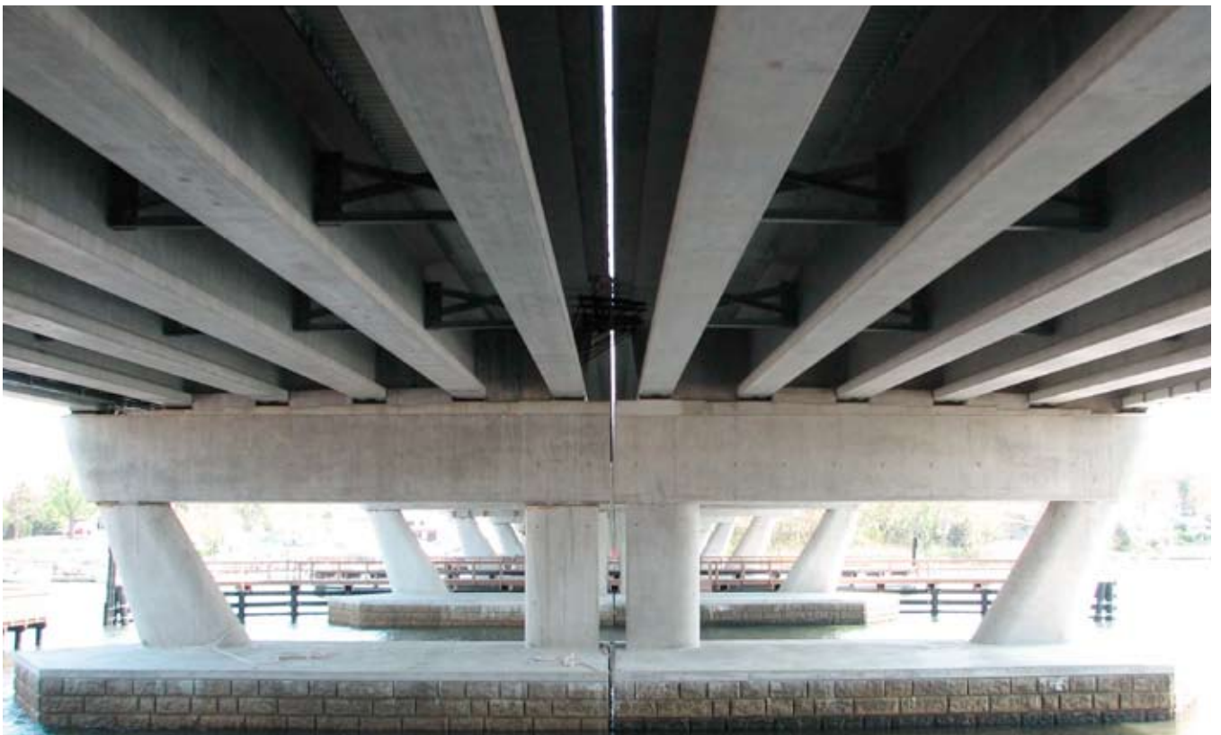
View of the precast elements and the underside of the bulb-tee girders.
